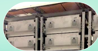
Fuel cell rack
